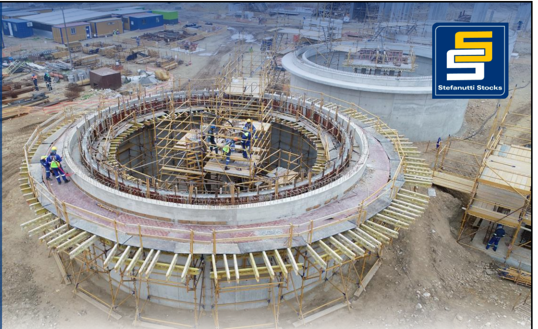
Paarl Waste Water Treatment Works, Drakenstein Municipality, Paarl, Western Cape
