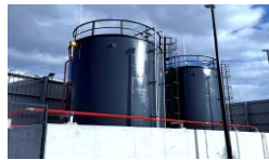
BULK FUEL STORAGE TANKS
