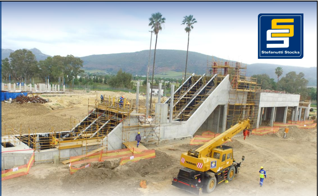
Inlet Works, Paarl Waste Water Treatment Plant, Drakenstein Municipality, Paarl, Western Cape
